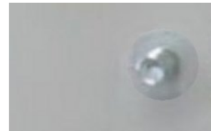
Fig. 20: Unmarked grounding stud
