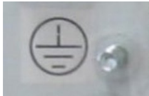
Fig. 25: Grounding stud marked with PE symbol
