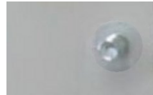
Fig. 26: Unmarked grounding stud
